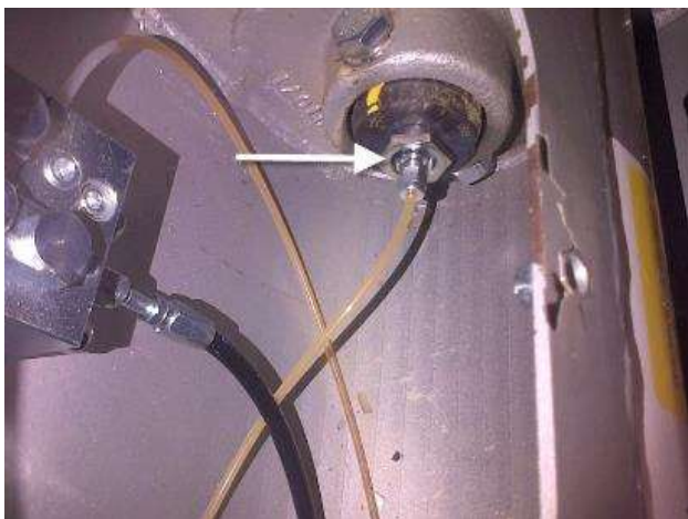
Connection points of the greasing circuit
